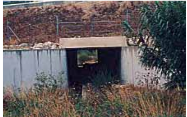
Photo 45 - LGV Méditerranée '52FF high-speed rail line (Bouches du Rhône department): type IIIc passage for beavers in the Durance river valley.
