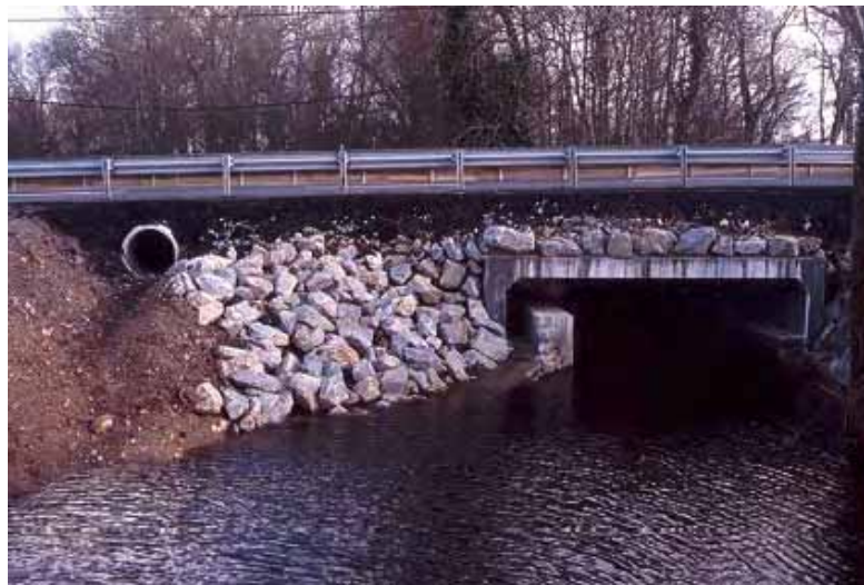
Photo 135 – Facility on Duchée bridge (Loire-Atlantique department): structure provided with a bench extending the river-banks and a pipe passage forming an emergency exit in the event of a flood – Source: X. Moyon - PRNB
