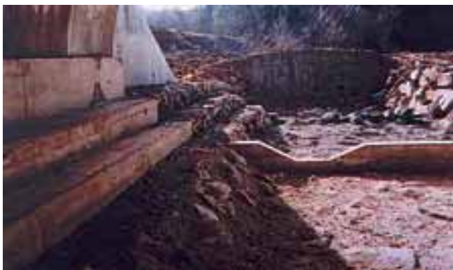
Photo 42 - RN 89 national road (Puy de Dôme department): type IIIb passage crossing the Clidane. Arched hydraulic structure ( \varnothing 5000 mm, length 75 m). Tiered river-banks (2 x 0.40 m wide ledges) are regularly used by the otter – Source : M. Owallar
