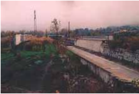
Photo 46 - A 43 motorway - SFTRF (Maurienne valley): St Bernard type III d canal bridge.
