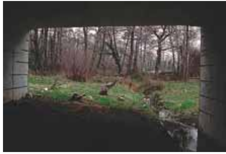
Photo 47 - A 89 motorway- ASF (Gironde department): mixed PI (hydraulic + fauna) underpass crossing the "Cholette". L = 30 m, l = 8 m, h = 4.3 m.
