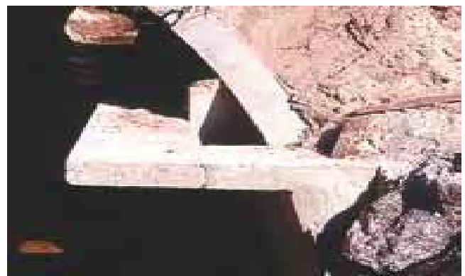
Photo 142 – Overspill from a road formation water treatment pond Source: Pascal Fournier
