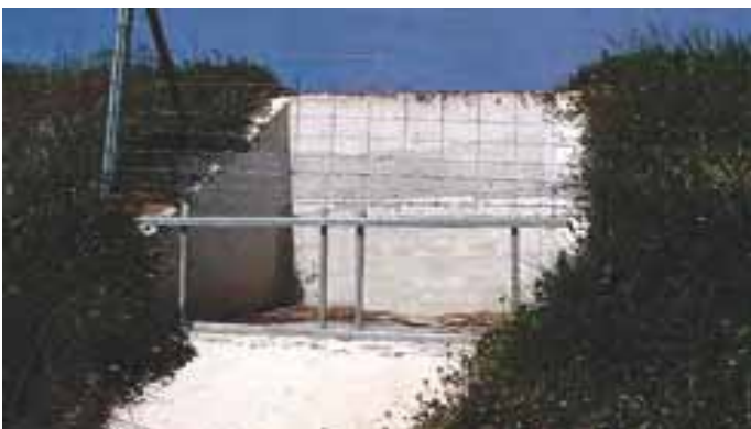
Photo 143 – Corbelling, but with the defect of not being connected to the watercourse bank – Source: Pascal Fournier
