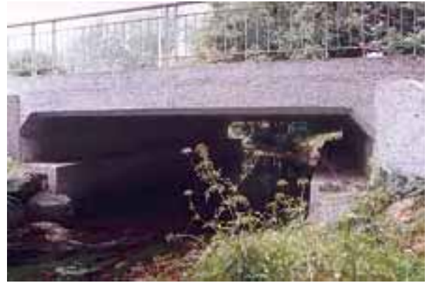
Photo 41 - RD 18 Sizun by-pass (Finistère department): type IIIb passage with ledge ( l = 0.75 m) on each bank.
