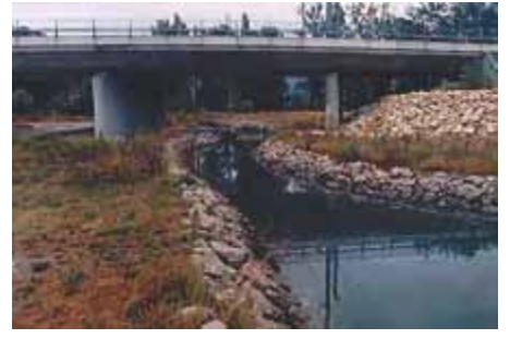
Photo 48 - LGV Méditerranée high-speed rail line. Type III d structure in the Durance river valley with extra width on both banks.
