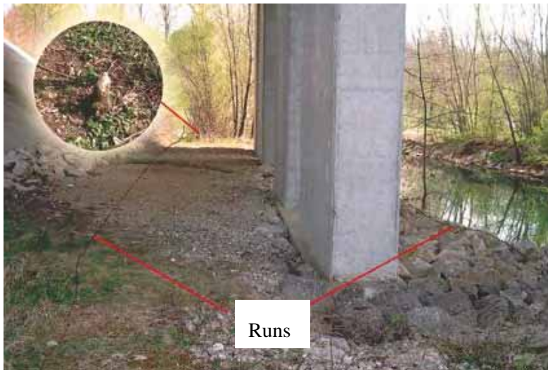
Photos 145 and 146 – Combined passage on A 40 motorway: structure patronised by the beaver. Two clues to presence indicate this usage: runs and felled trees.
