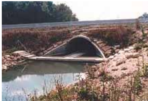
Photos 56 and 57 – Hydraulic passages unsuitable for land and fish fauna
